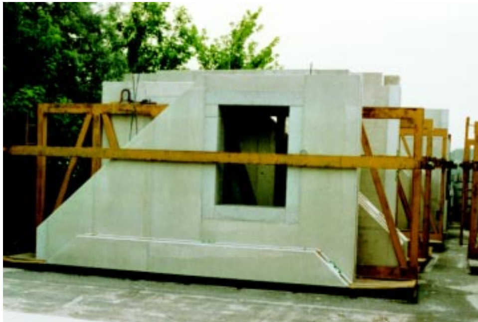
Figure 8.17 Racks with custom panels awaiting delivery.
