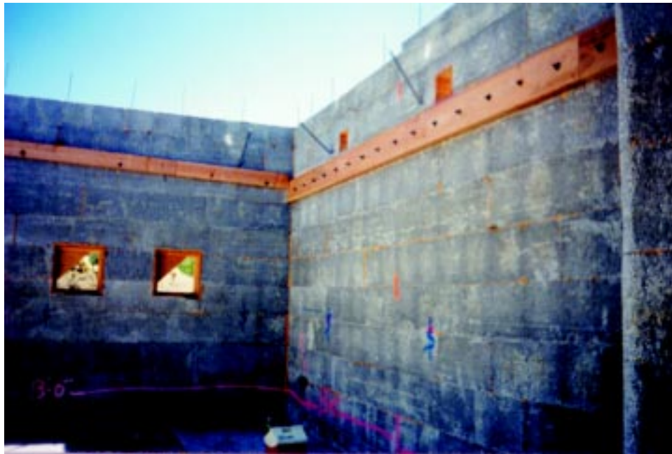
Figure 4.2 Ledgers with anchor bolts held in place with all thread rod prior to grouting of wall.
