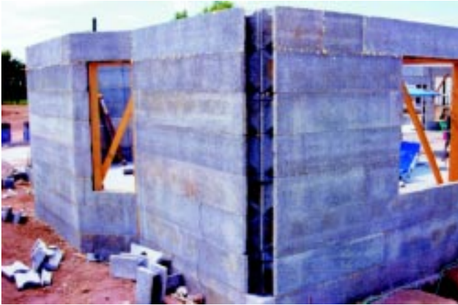
Figure 5.3 Ready for installation of corner element. Horizontal and vertical rebar in place.
