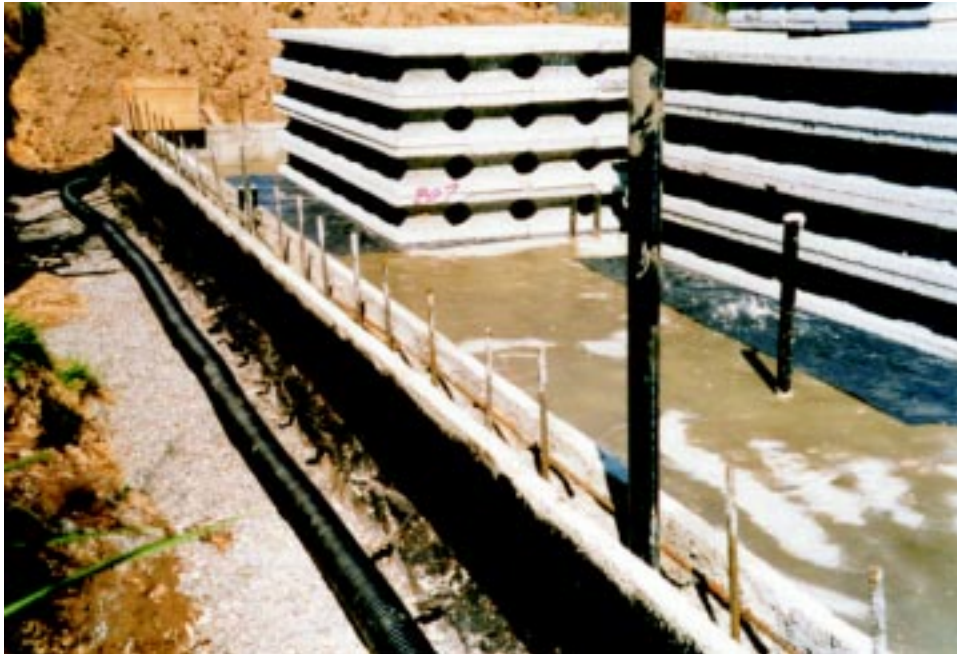
Figure 3.8 First course of elements, starter bars and first horizontal rebar in place.
