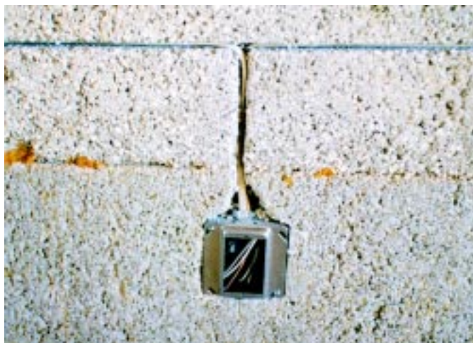
Figure A.6 Closeup of electrical box.
